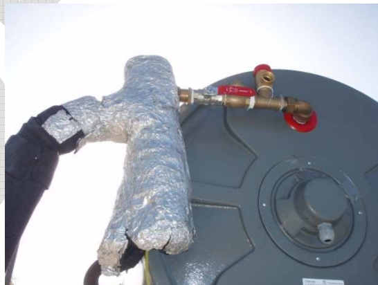
Fig. 4: hot water outlet
